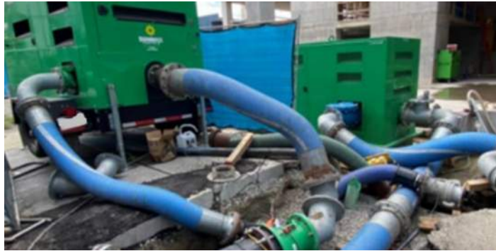
Figure 4.1.3-17: Example of temporary Pumping Skids and Electrical Generation
