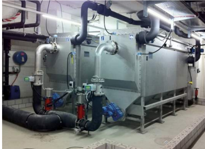
Figure 4.1.3-5A: Example photo of Huber (represented by Noventa) sewer water heat exchange system
