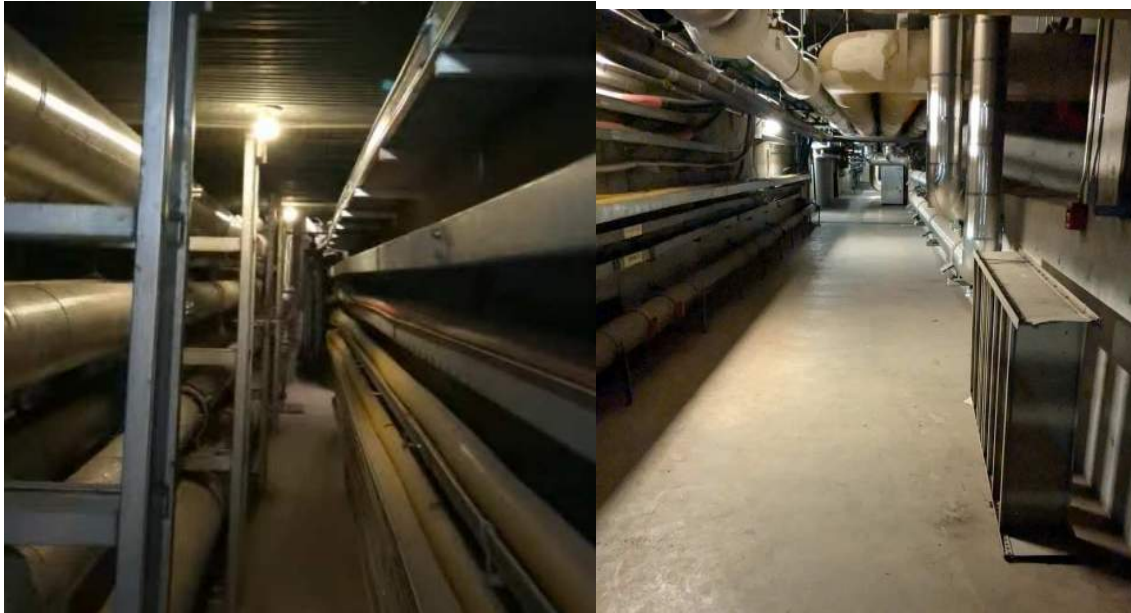
Fig B-11-5: I-Wing(left) and J-Wing(right) Utility Tunnel/Corridors
