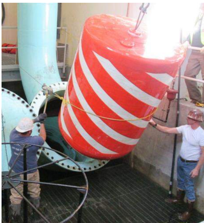
Figure 3-26. Loading a pig into the pig launcher, courtesy of Cornell University
