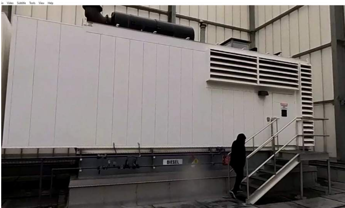
Figure 1.1.1.1 Photo of existing rooftop generator.
