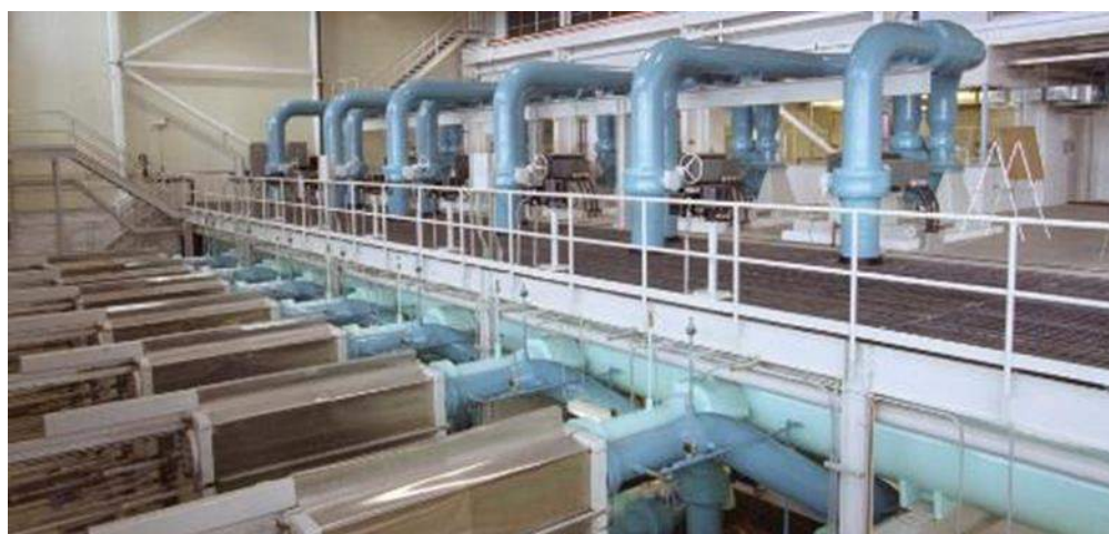
Figure 3-19. Photo of the 7 Lake Source Cooling heat exchangers (51 MW total), courtesy of Cornell University.
