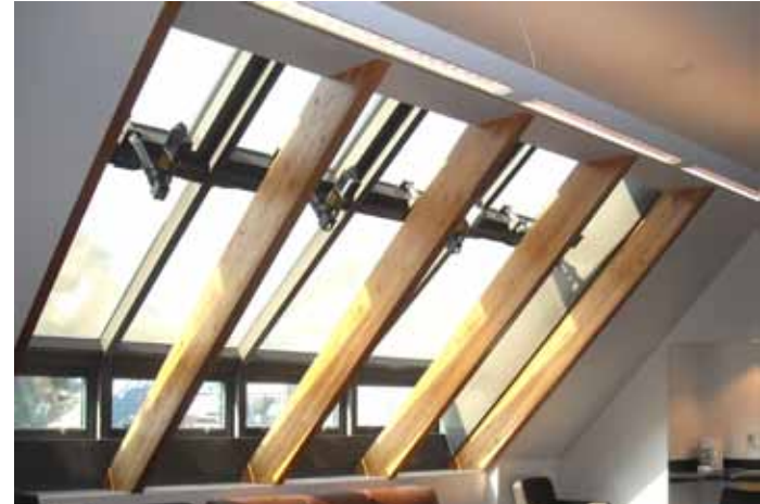
Automatically controlled naturally ventilating windows
